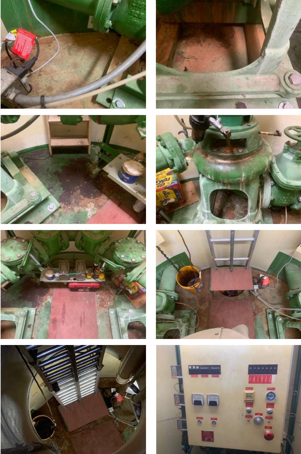
Figure 4 Lincoln Street Sewer Lift Station
