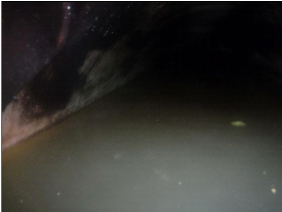
Monitored Influent Pipe
