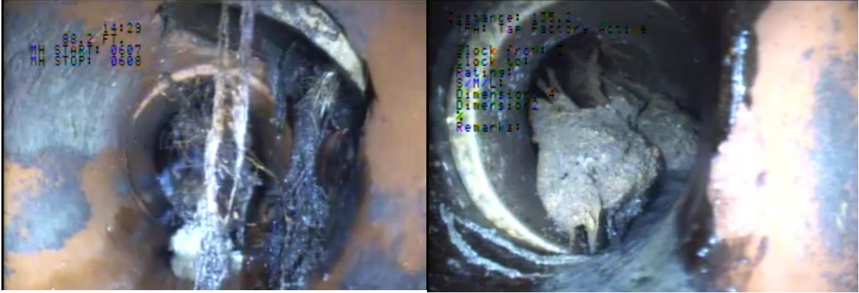
Figure 3 Typical O&M Defects from City's CCTV Inspections
