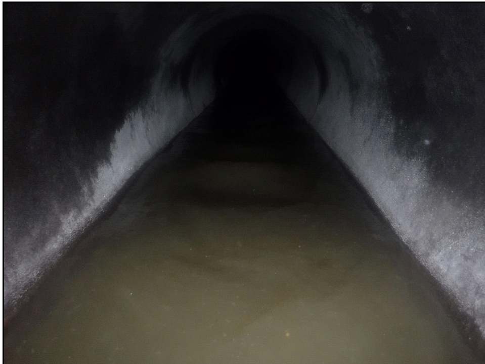
Monitored Influent Pipe
