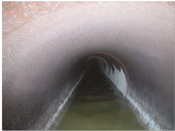
Monitored West Influent Pipe
