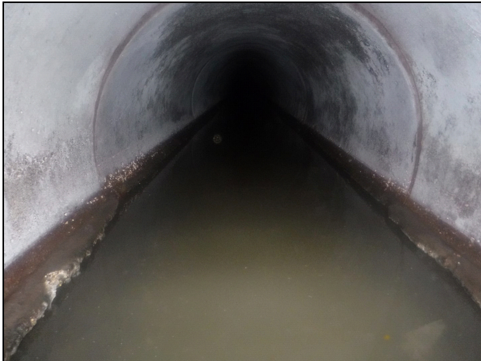
Monitored Influent Pipe
