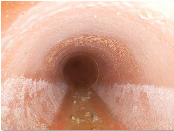
North Influent Pipe
