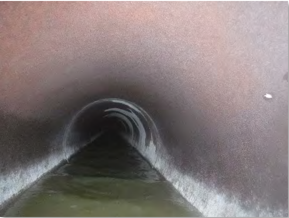
Monitored West Influent Pipe
